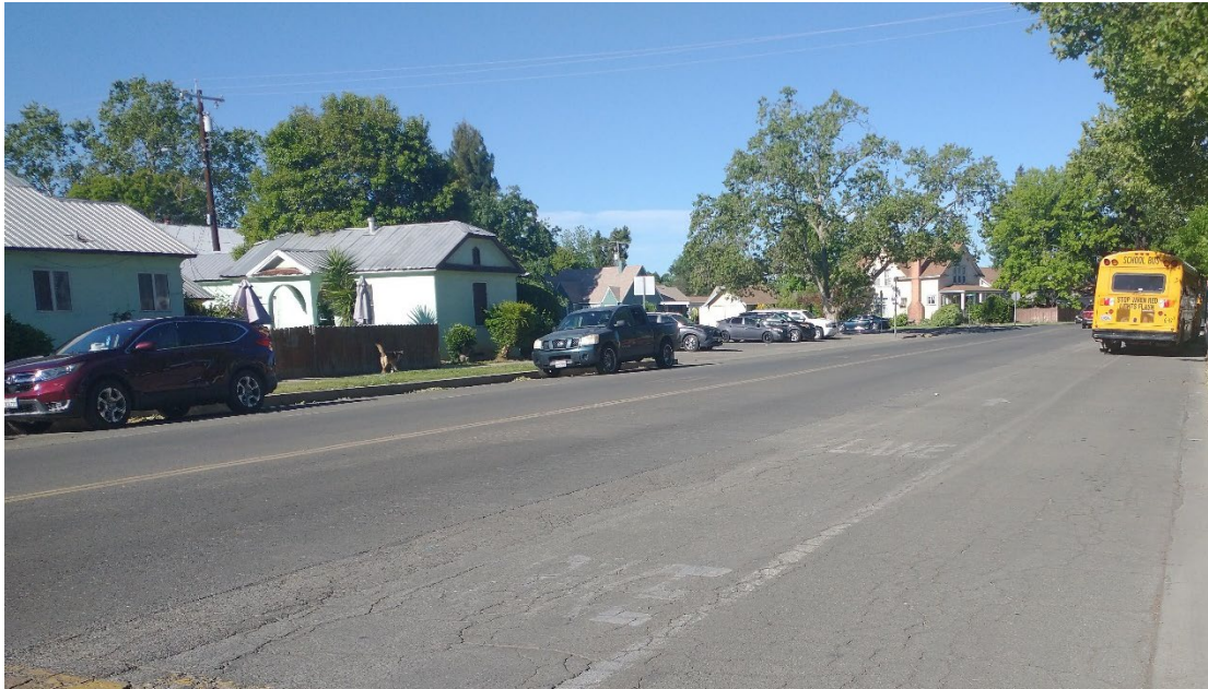
Faded bike lane on Magnolia Street
